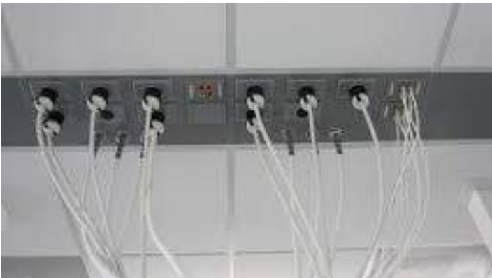
Ceiling Service Panels
